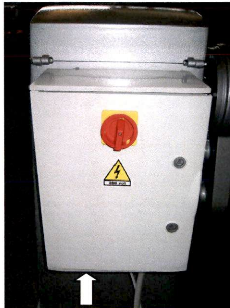
Electric supply inlet
